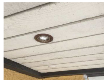
Figure E.40: FCO, mounted in ceiling, UH: 0% UL: 0%, ULR: 0%
