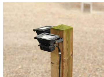
Figure E.28: LED spotlight as uplight below a tree, nonFCO. UH: 100%, ULR: 100%.
