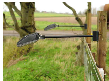
Figure E.27: Downlights for sign. Installed correct, as here, these fixtures are FCO. UH: 0%, UL: 0%, ULR: 0%
